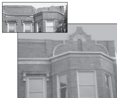
The crumbling facade on this apartment building at 4343 S. Michigan Avenue was restored to its original state through the Troubled Buildings Initiative.
