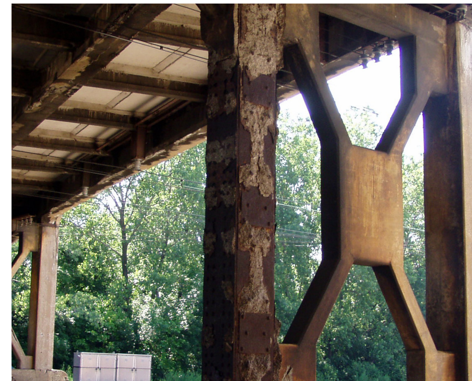
Pier 1 with cracked, delaminated, and spalled encasement
