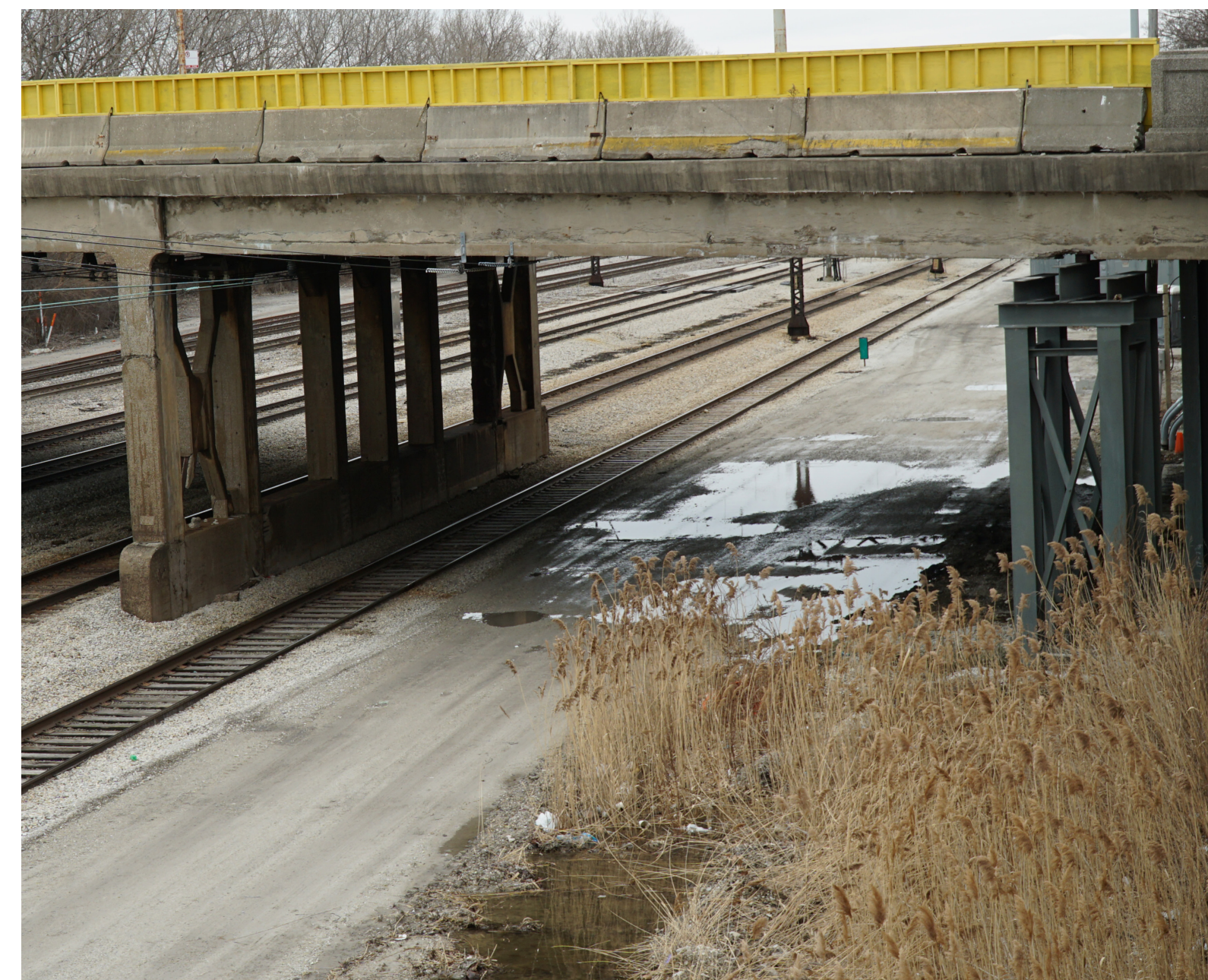
Temporary shoring has been installed in front of the west abutment to support the girders
