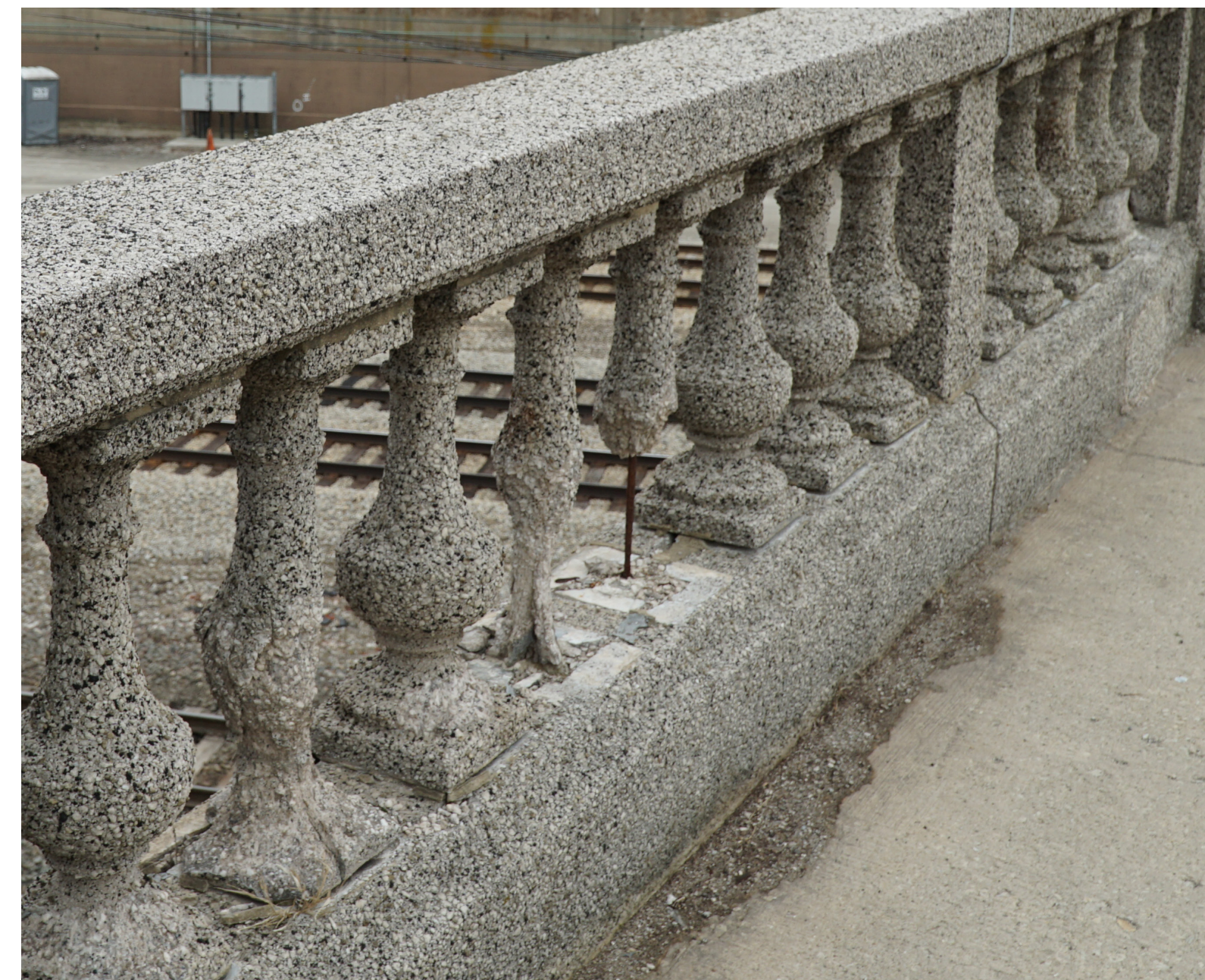
The south side railing has sections of potentially dangerous openings
