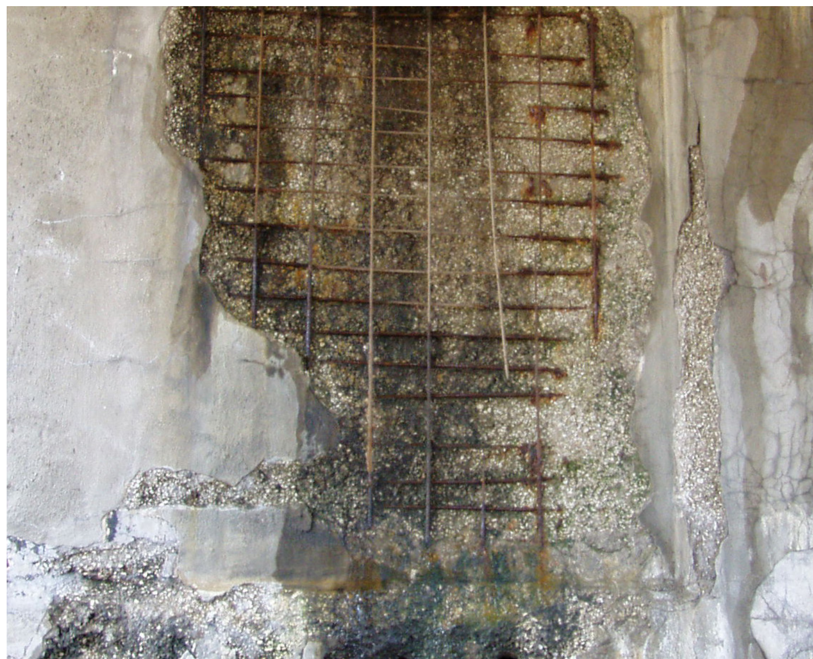
The west abutment has large areas of spalling, cracking, and delamination with exposed broken reinforcing steel
