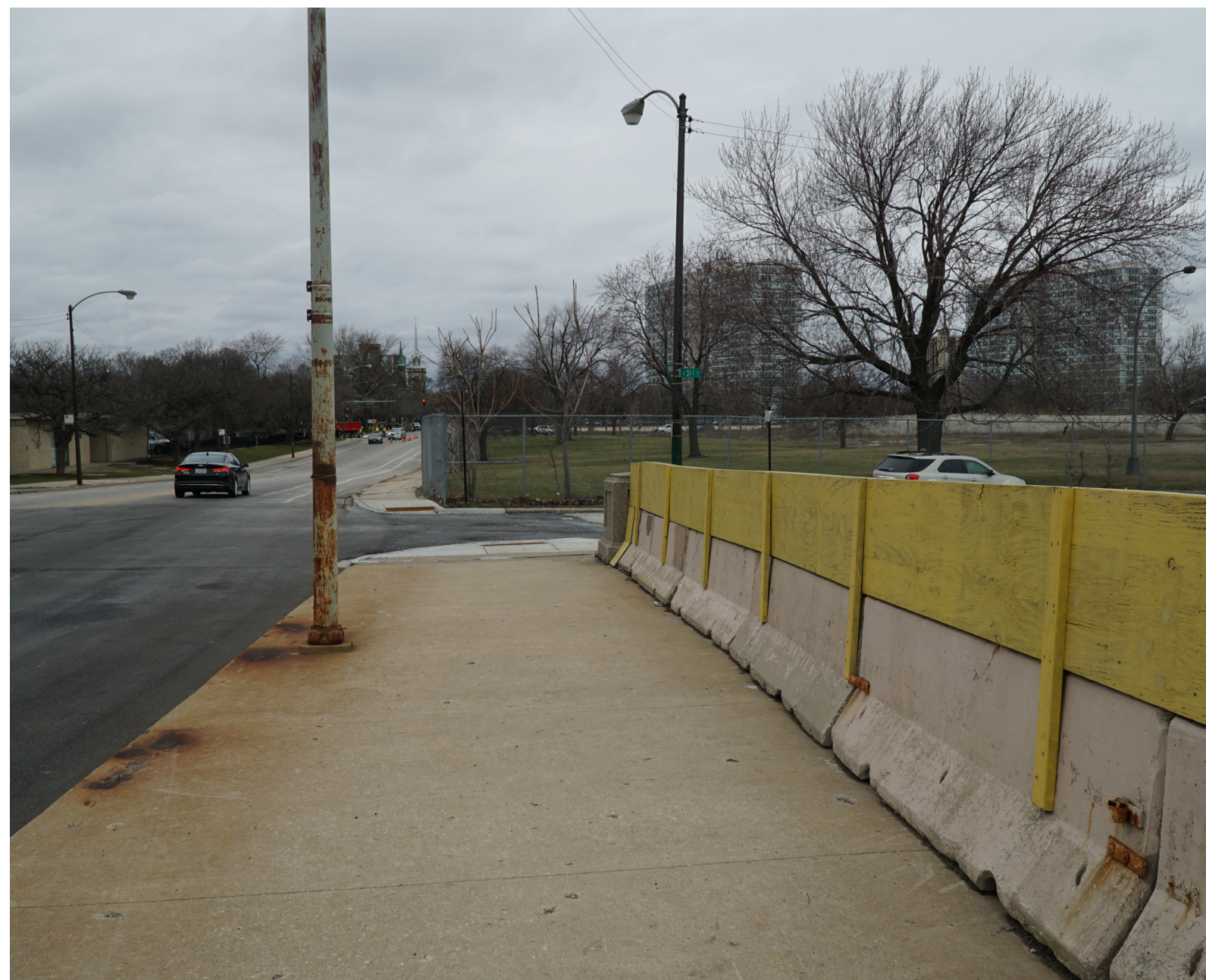
The north side railing has been replaced with temporary concrete barrier over the entire length of the bridge
