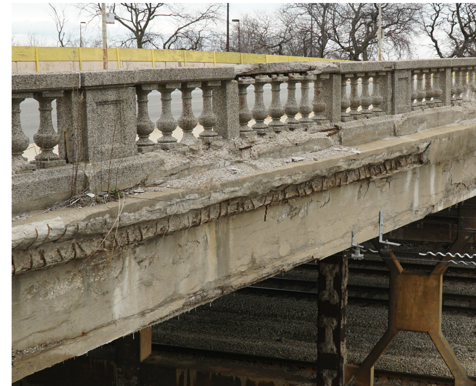
South fascia with cracked and loose concrete encasement
