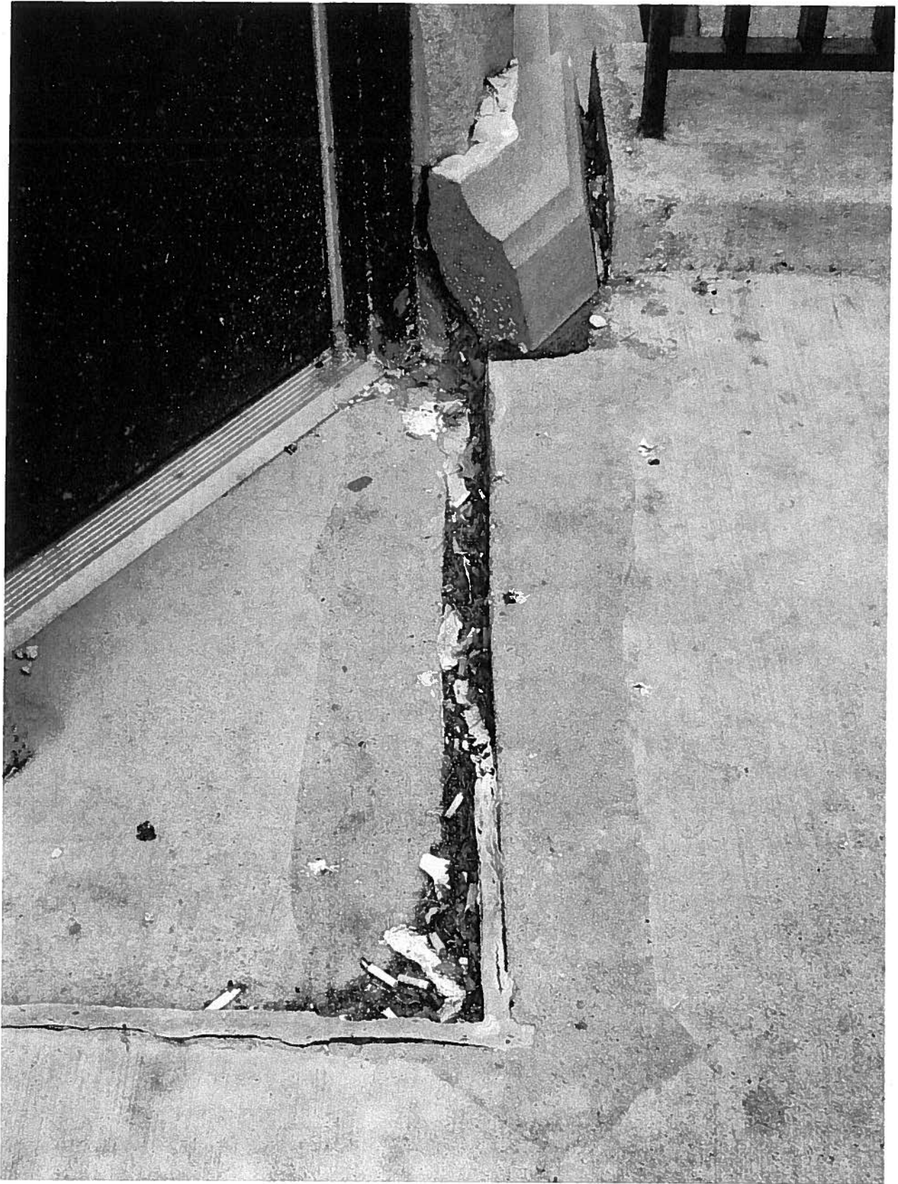
Separation at entrance to bridge house.
