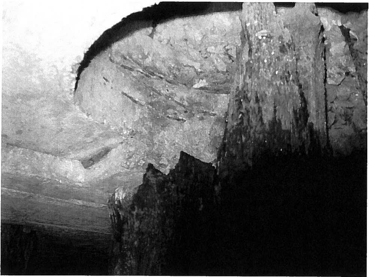
Timber pile 6G near the northeast corner of the Madison Street Bridge House. Note that the timber pile no longer touches the pile cap.
