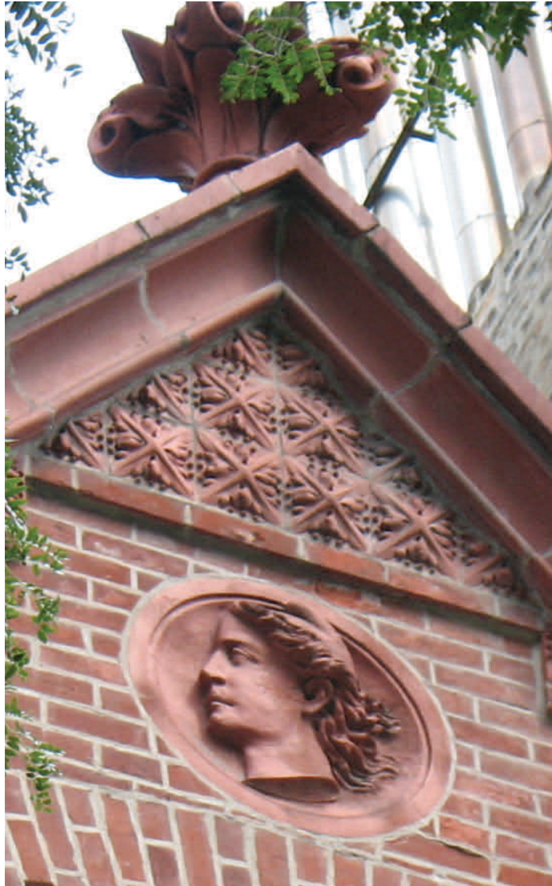
A close-up view of the Warner House's roofline gable with its terra-cotta "cameo" medallion, foliate ornament and Gothic-style finial.
