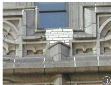
Inappropriate replacement of stone
