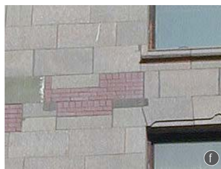
Inappropriate replacement of stone
