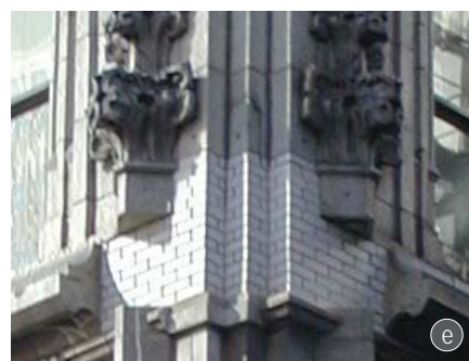
Inappropriate replacement of terra cotta
