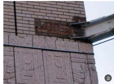
Inappropriate facade maintenance
