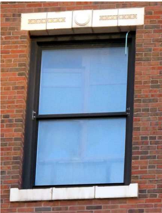
The window openings on floors three to six (above) from 1911 include white terra-cotta lintels with simple geometric decoration; sills are plain white terra cotta.
