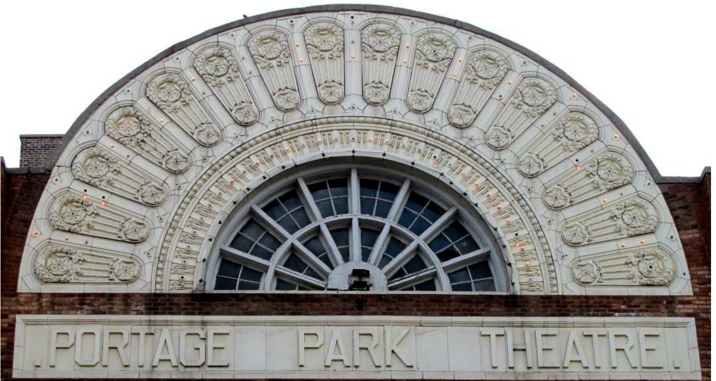
Cream-colored terra cotta decorates the façade of the Portage Theater with motifs derived from classical architecture. An image of a lyre (top left) rendered in terra cotta is repeated along the building's cornice and brick piers (top right) are accented along their length green tiles. Much of the terra cotta is fitted with sockets for incandescent lighting. The prominent arch and fanlight (bottom) at the top of the building makes the building a prominent visual feature of the "Six Corners" neighborhood commercial district.
