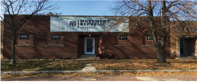
The use of traditional brick and stone masonry is prevalent and should be retained and repaired.
