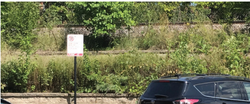
Example of naturalized landscape with modular segmented retaining wall along Union Pacific Railroad embankment.
