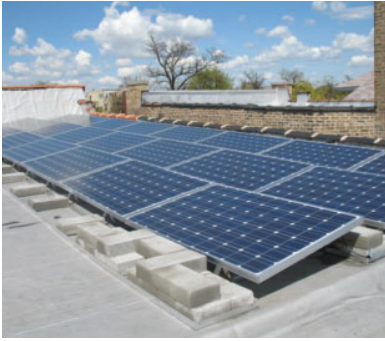
An example of a ballasted (non-penetrating) solar PV system. Here, the PV panels are not physically connected to the roof. Cinder blocks are used as ballasting means to secure the system to the roof.
