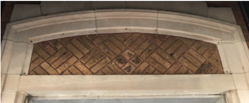
The combination of cast stone and brick inserts are also prevalent and should be retained and repaired.
