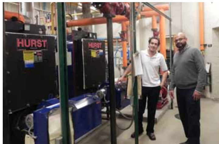
Above left: Quigley Building. Above (left to right): Nick Fernandez – RE Data Administrator and Jacob Preciado – Facilities Construction Manager.
