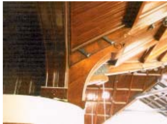
Middle: Scrollwork detail on the roof trusswork. The roof is made from red oak and chiefly supported by large concrete columns.
