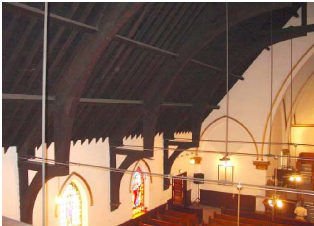
The main sanctuary of the Truevine Missionary Baptist Church Building has a fine open-truss wooden ceiling.
