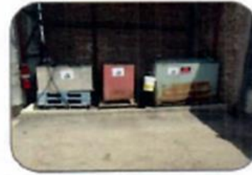
6-1. Fluids Secondary Containment and Precipitation Protection
