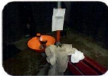
3-9. 15-Minute Eye Wash Station
