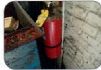
3-10. Fire Extinguisher (Tag Visible)
