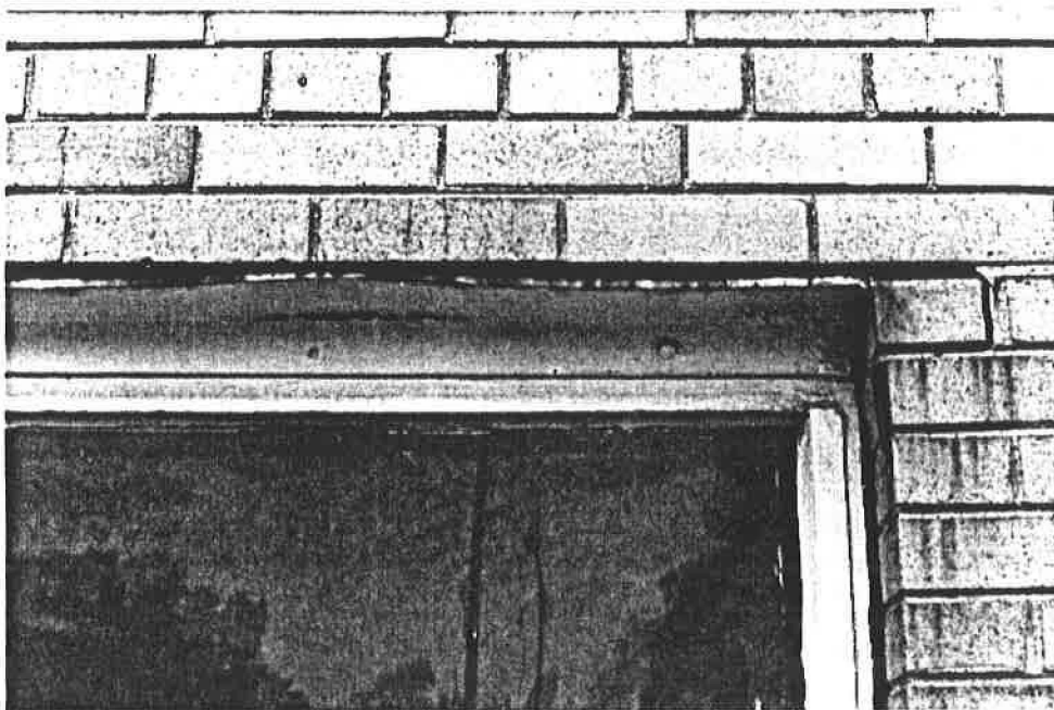
PHOTO S-6 Buckled lintel flanges (close-up).
