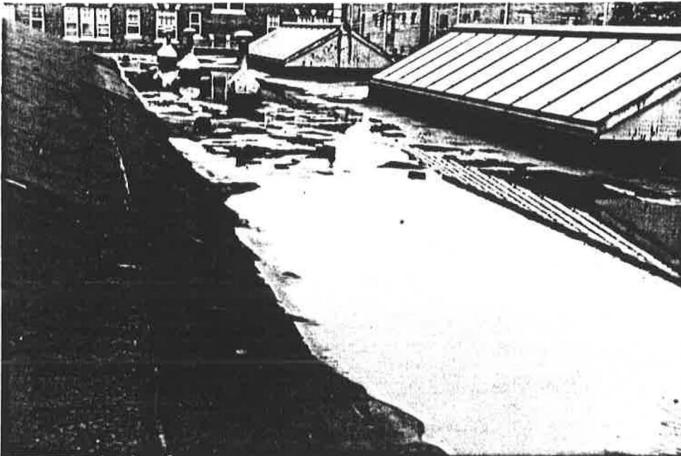
PHOTO A-5 Ponding water on roof and skylights.
