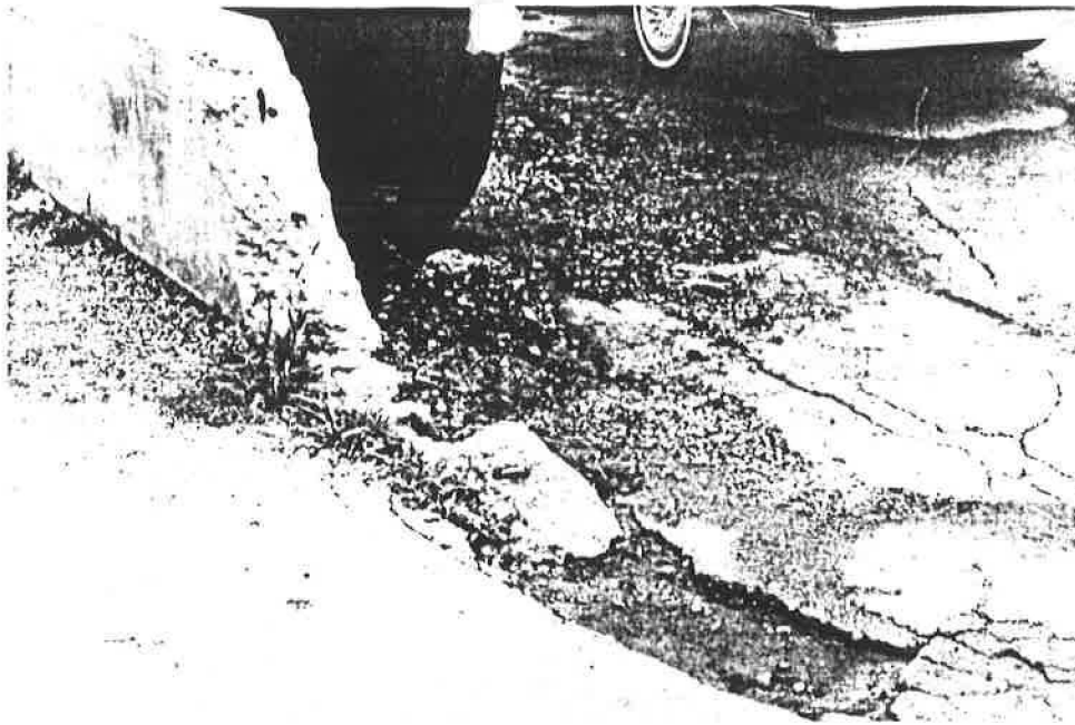
PHOTO S-12 Deteriorated retaining wall near service addition.
