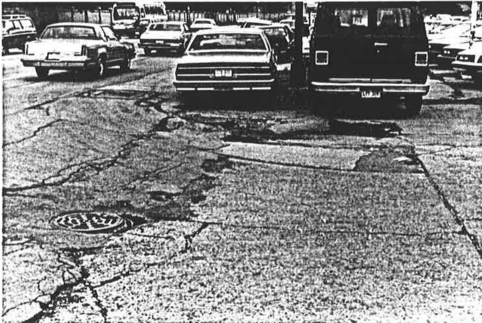
PHOTO C-2 Aged and deteriorated paving.
