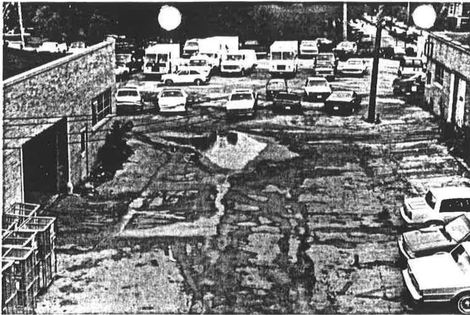
PHOTO C-1 Ponding storm water.
