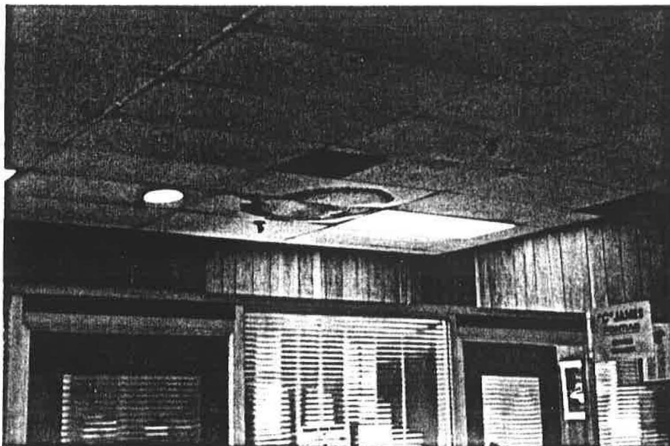
PHOTO A-6 Damaged ceiling tiles.
