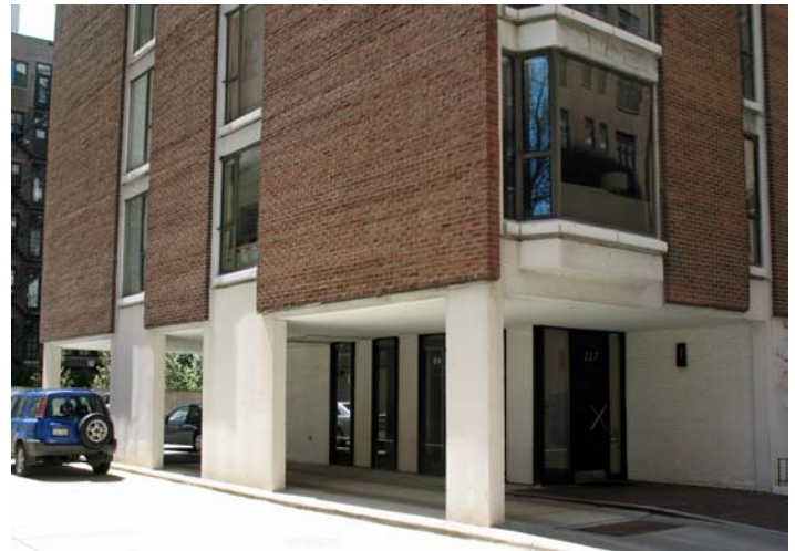
The base of the building with recessed lobby and exposed concrete structure.
