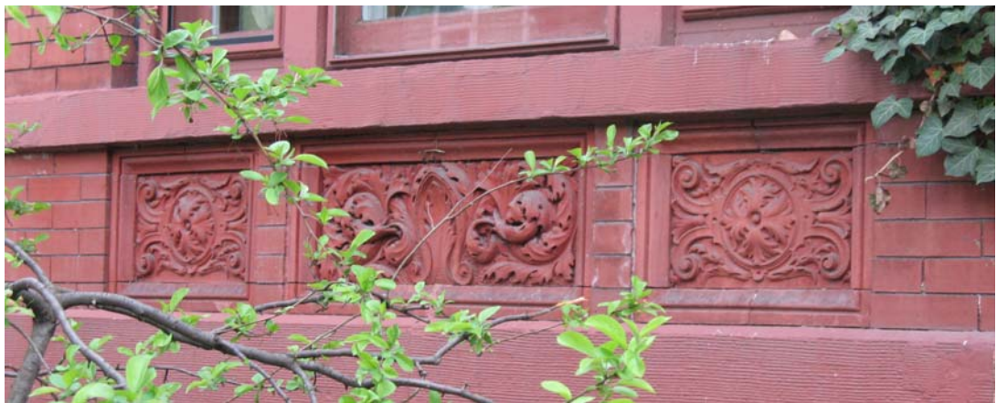
The building's projecting front bay combines a Chicago-style window and round-arched, stained-glass-filled transom with bulls-eye-detailed window sash and terra-cotta ornament.
