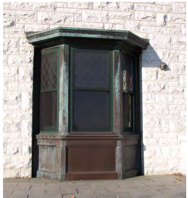
Top: The Wheeler House's front entrance, with its carved marble surround detailed with a Classical-style foliate garland. Bottom left: The front porch has both massive rusticated-marble piers and more delicate, smoothly-finished Classical-style columns. Bottom right: A copper bay on the house's east façade.
