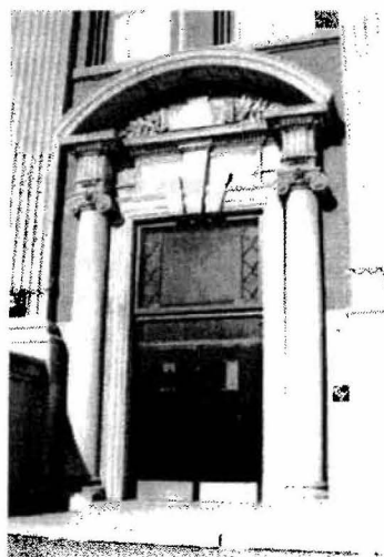
Above: One of the three elaborate archways on the south elevation of the school. Doors have stone columns on either side with transoms overhead topped by decorative carved stone lintels.
