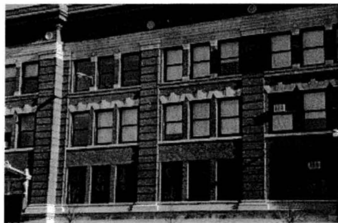
Above: Cut stone lintels with raised keystones embellish the second-floor windows of the school.
