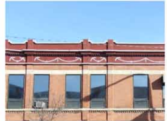
Inappropriately proportioned, mirror glass windows
