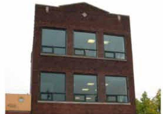
Inappropriately proportioned windows
