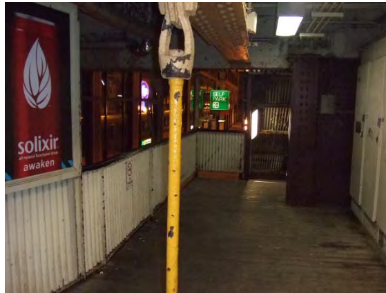
LBP-15: HANGER SUPPORT ON LOWER LEVEL OF RANDOLPH ST. STATION ABOVE STREET.
