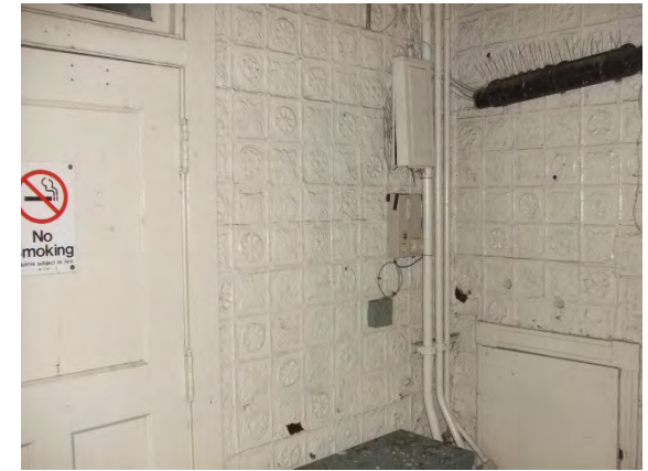
LBP-07: LOWER LEVEL OF MADISON ST. STATION ABOVE STREET. TEXTURED PAINT ON OLD STATION HOUSE.
