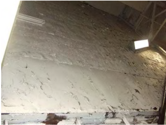
LBP-04: LOWER LEVEL OF MADISON ST. STATION ABOVE STREET. CORRUGATED METAL ON OLD MADISON ST. STATION.
