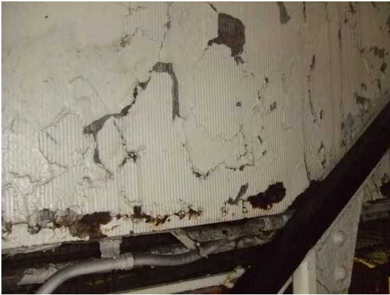
LBP-03: LOWER LEVEL OF MADISON ST. STATION ABOVE STREET. CORRUGATED METAL ON OLD MADISON ST. STATION.
