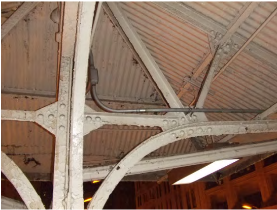
LBP-05: CANOPY SUPPORTS ON PLATFORM OF MADISON ST. STATION. (THIS WAS THE TYPE OF STRUCTURE FOR RANDOLPH ST. STATION LBP-13 & 14.)
