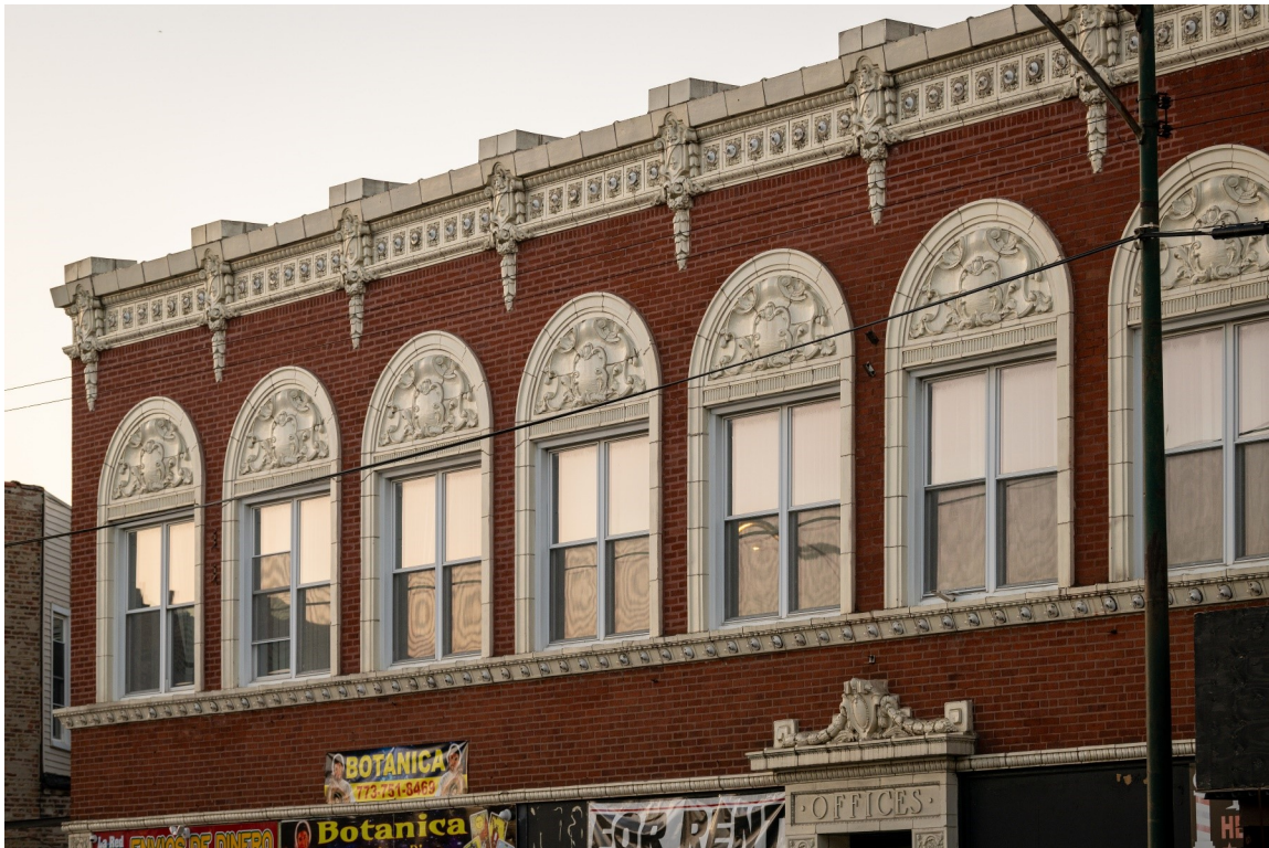
Ornamental terra cotta details include sculptural eagles (above), cartouches and festoons (below) that are influenced by Beaux Arts style of architecture.
