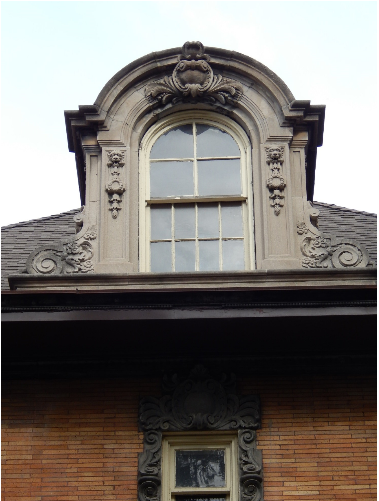
A photograph of some of the elaborate stone decoration that ornaments the Daniel O. Hill House.
