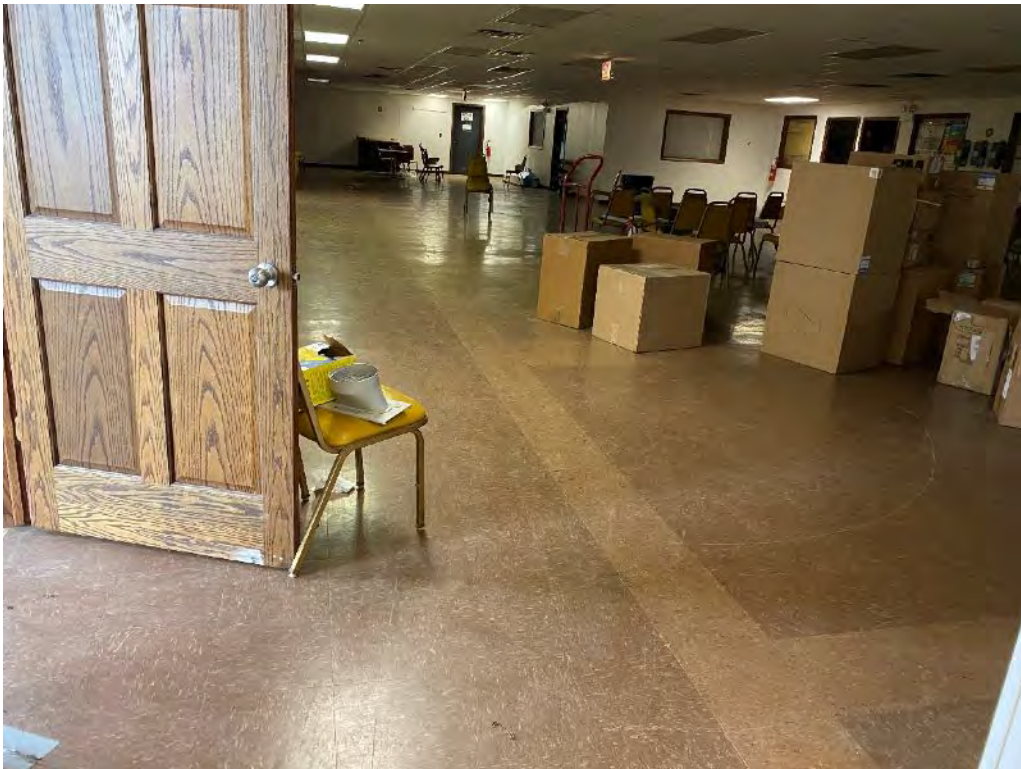
Asbestos Containing 12"x12" Brown w/ Beige Streaks Floor Tile and Associated Mastic – Main Office
