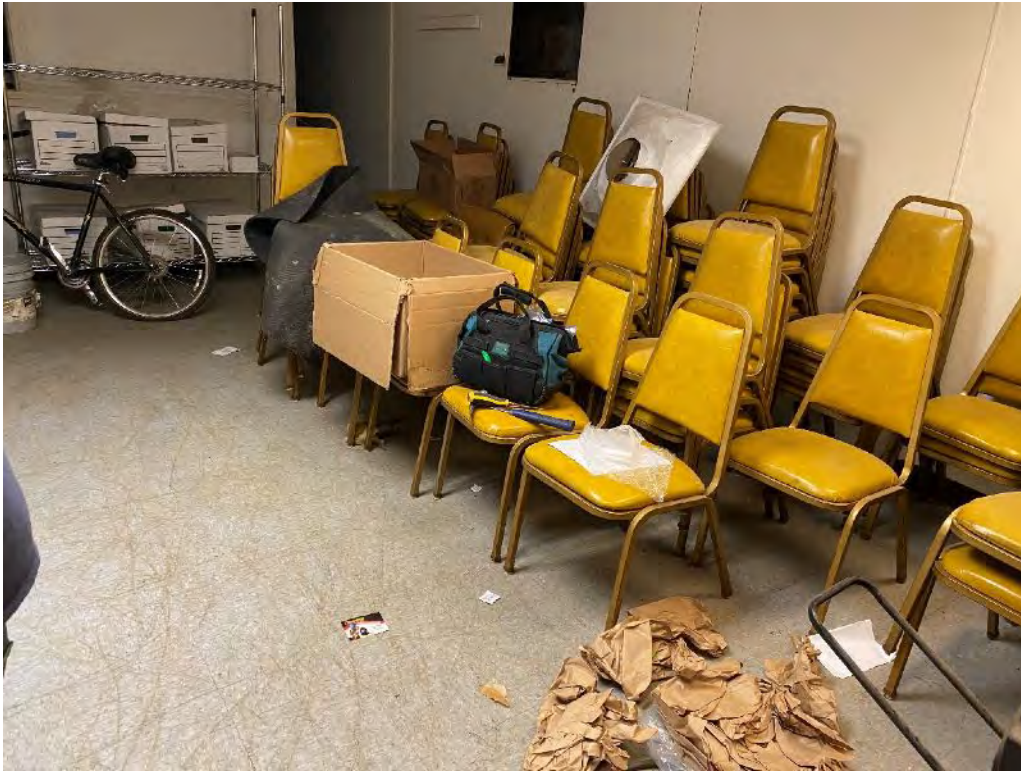
Asbestos Containing Residual Black Mastic assoc. w/ 12"x12" Gray Mottled Floor Tile – Main Office
