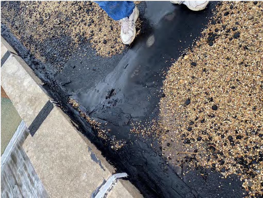
Asbestos Containing Roof Flashing – General Metals
