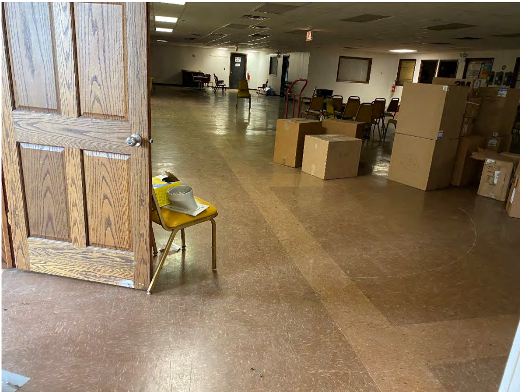
Asbestos Containing 12"x12" Brown w/ Beige Streaks Floor Tile and Associated Mastic – Main Office
