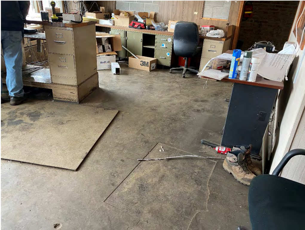
Asbestos Containing 12"x12" Black Floor Tile and Associated Mastic – Main Office
