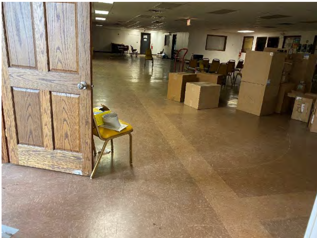
Asbestos Containing 12"x12" Brown w/ Beige Streaks Floor Tile and Associated Mastic – Main Office
