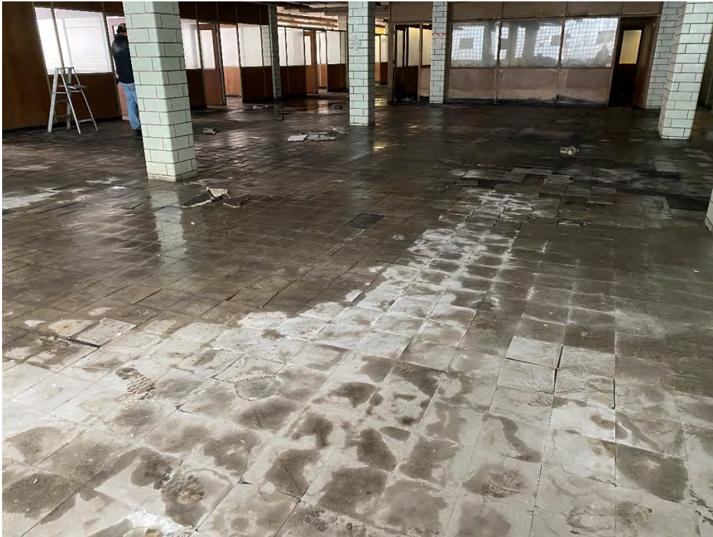
Asbestos Containing 9"x9" Gray Floor Tile and Associated Mastic – General Metals
