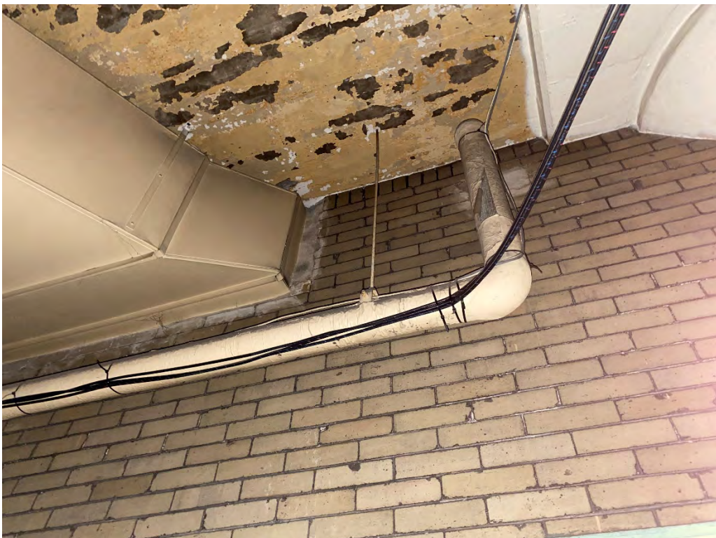
Asbestos Containing Fittings on Fiberglass – General Metals
