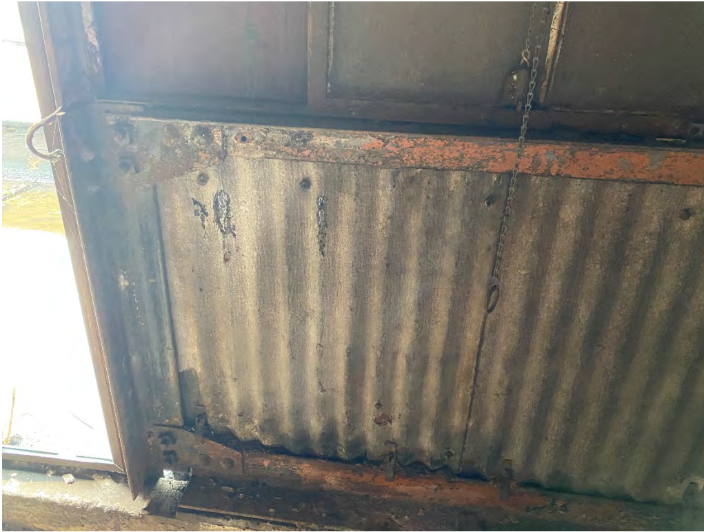
Asbestos Containing Tar Like Coating on Steel Panels – General Metals
