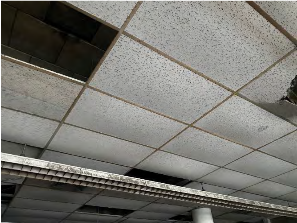
Asbestos Containing 2'x4' Lengthwise Fissure Lay In Ceiling Tile – General Metals
