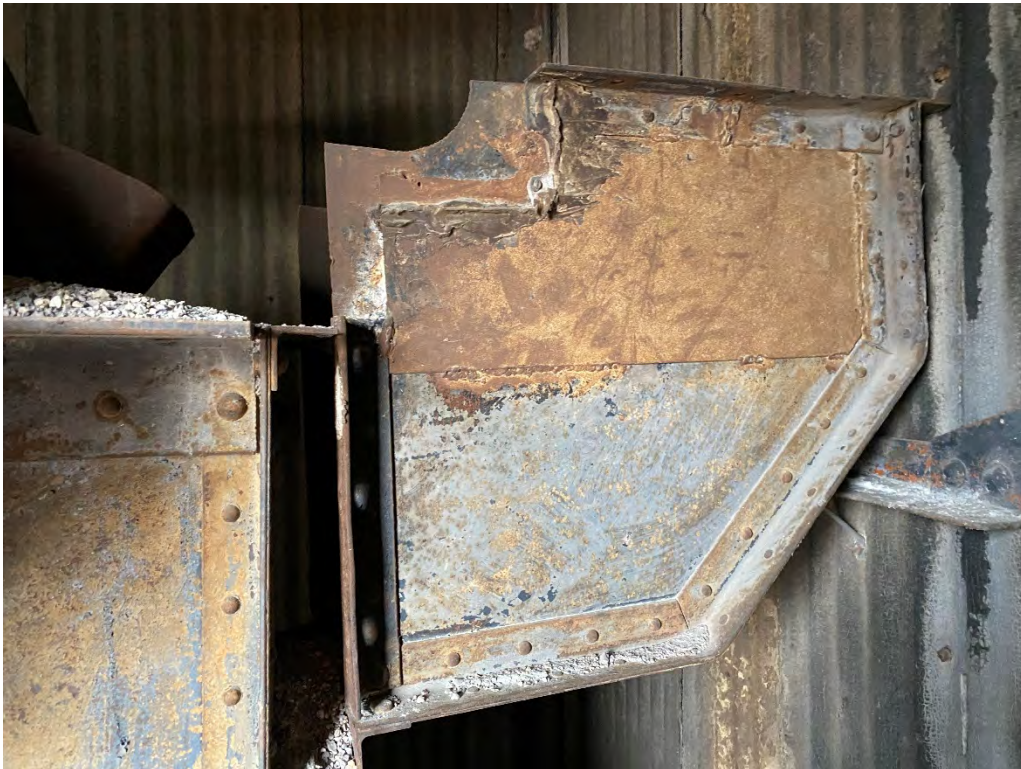
Asbestos Containing Caulk on Mechanical Equipment – General Metals
