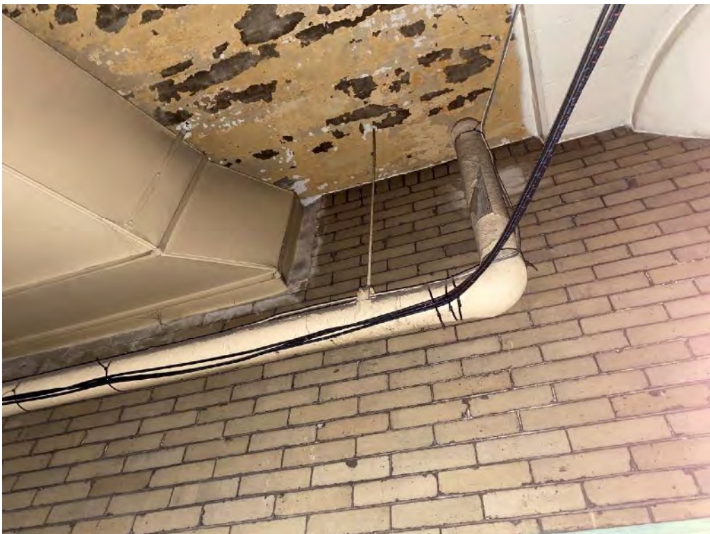
Asbestos Containing Fittings on Fiberglass – General Metals
