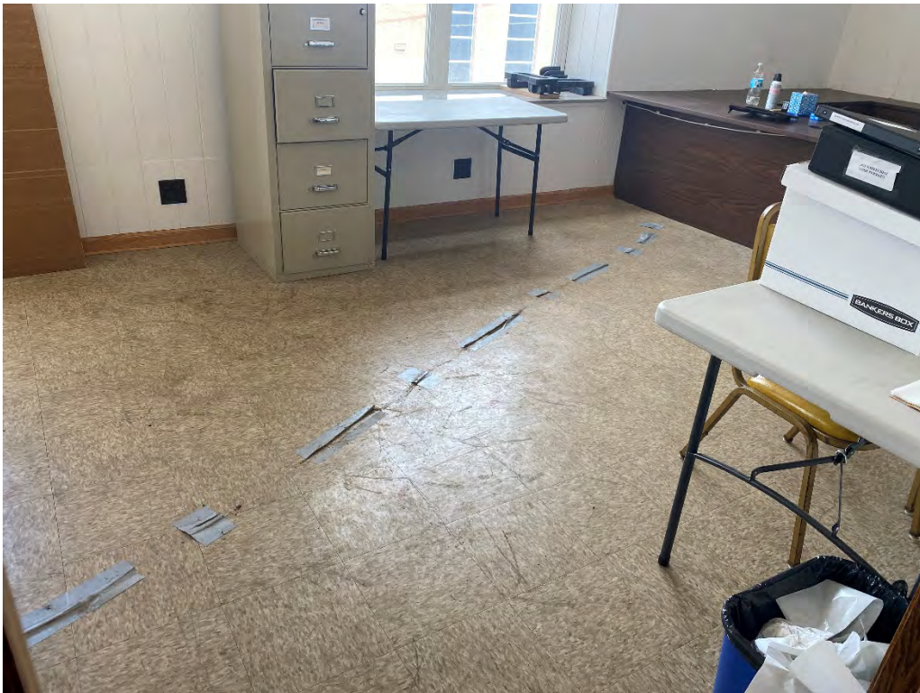
Asbestos Containing Black Mastic assoc. w/ 12"x12" Beige Mottled Floor Tile – Main Office
