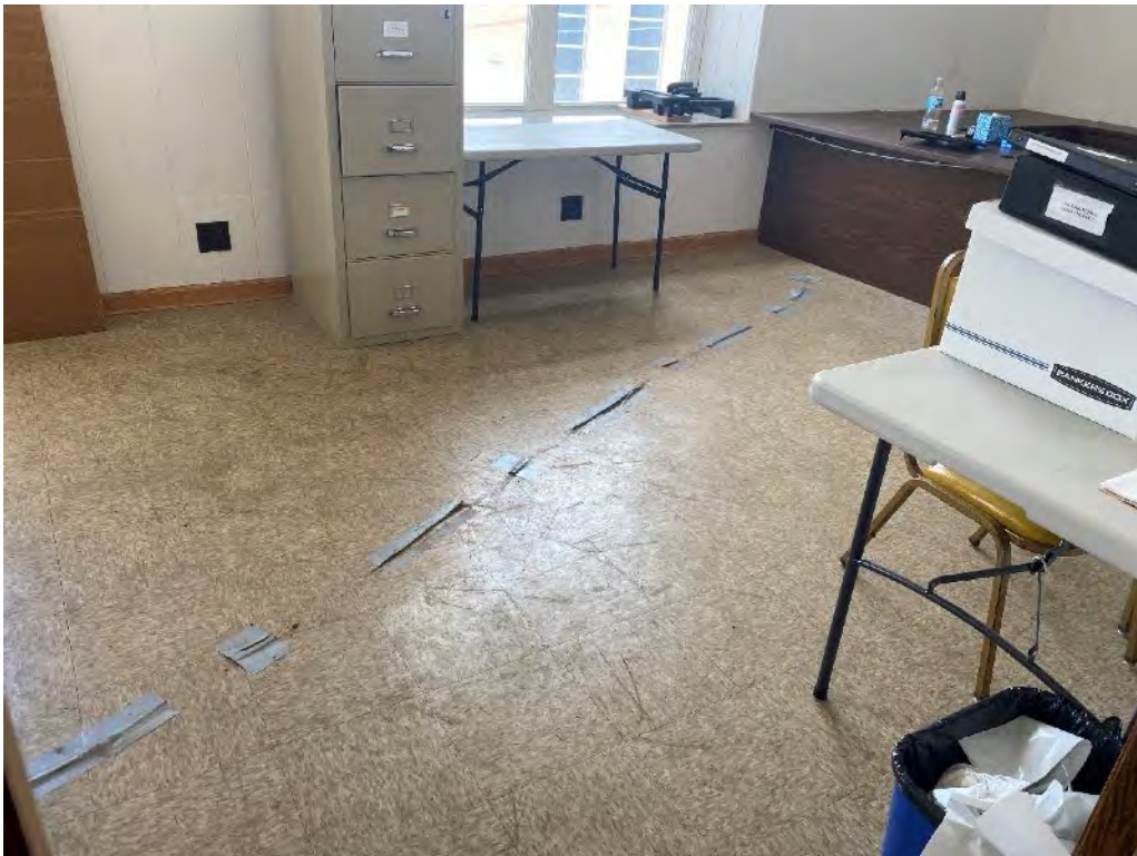
Asbestos Containing Black Mastic assoc. w/ 12"x12" Beige Mottled Floor Tile – Main Office
