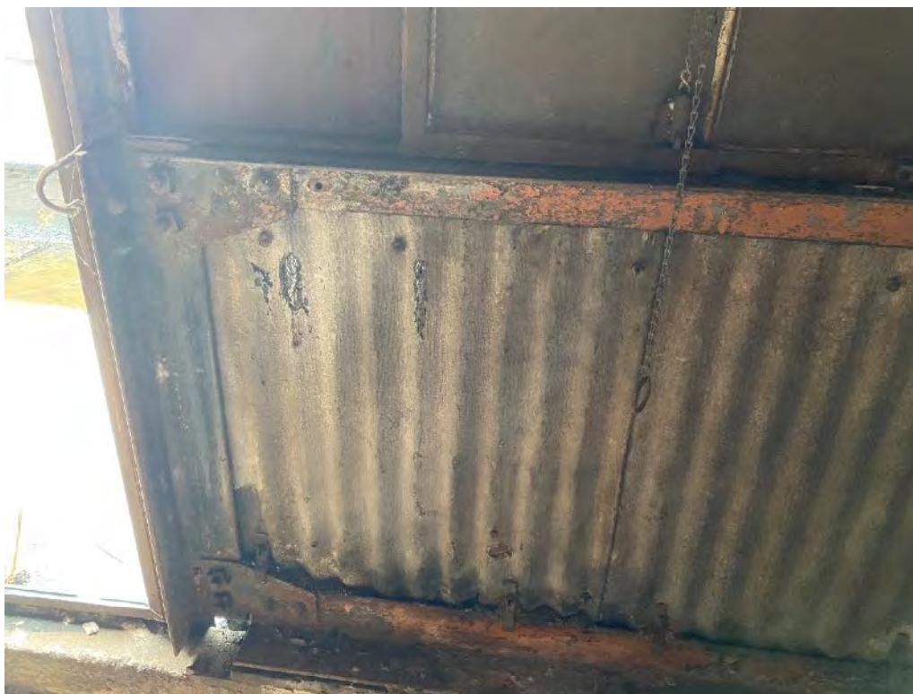
Asbestos Containing Tar Like Coating on Steel Panels – General Metals
