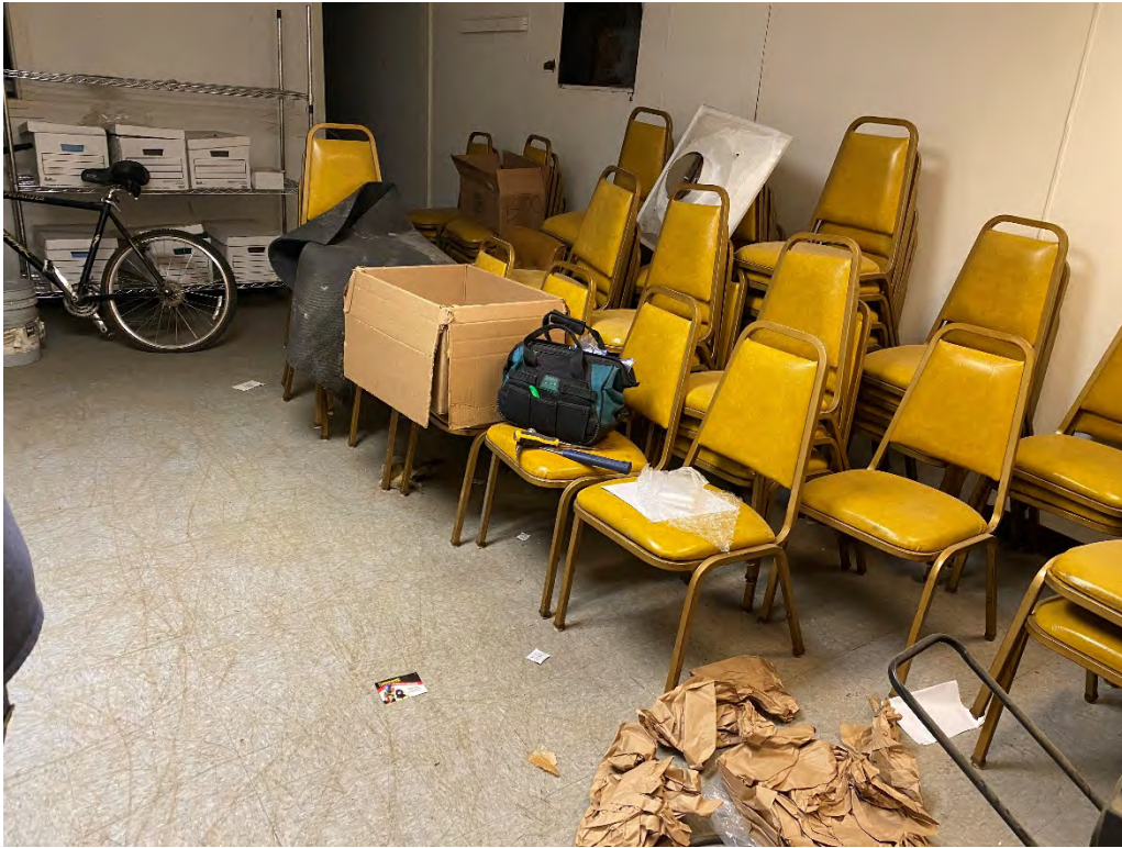
Asbestos Containing Residual Black Mastic assoc. w/ 12"x12" Gray Mottled Floor Tile – Main Office
