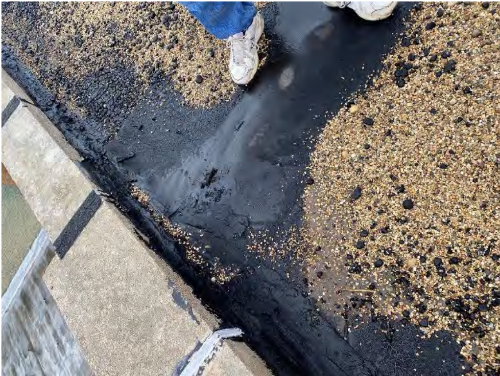
Asbestos Containing Roof Flashing – General Metals
