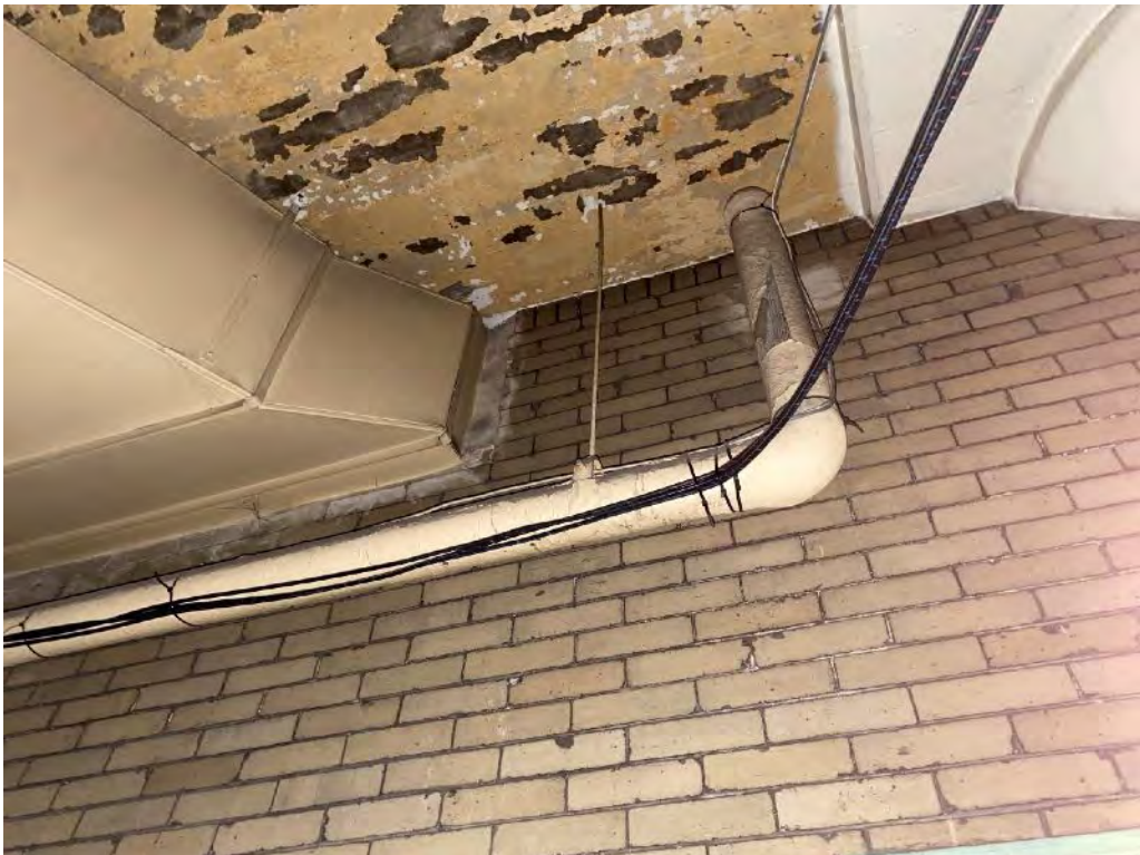
Asbestos Containing Fittings on Fiberglass – General Metals
