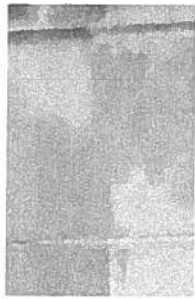
Roughly 15 inch crack
