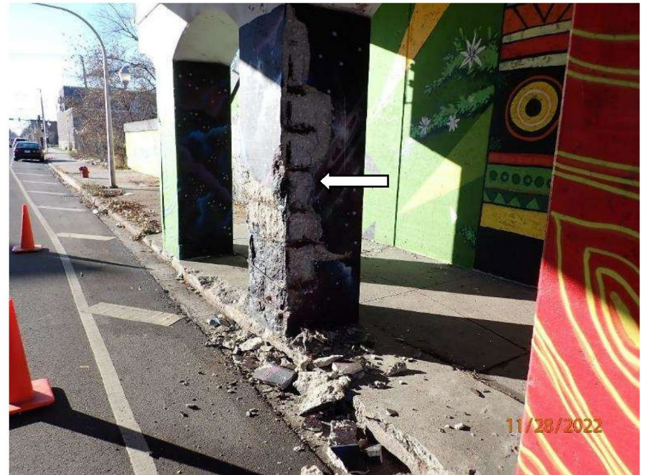
Photo 24: Concrete spalls on Column 2 of Pier 1, looking southwest
