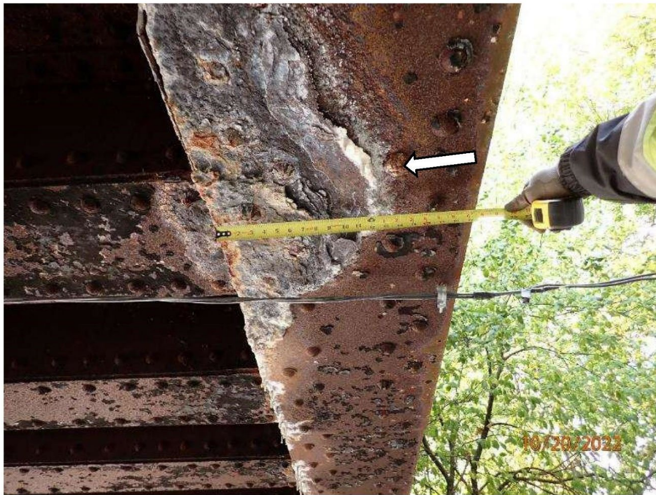
Photo 15: Corrosion on north girder over southbound lane, looking west
