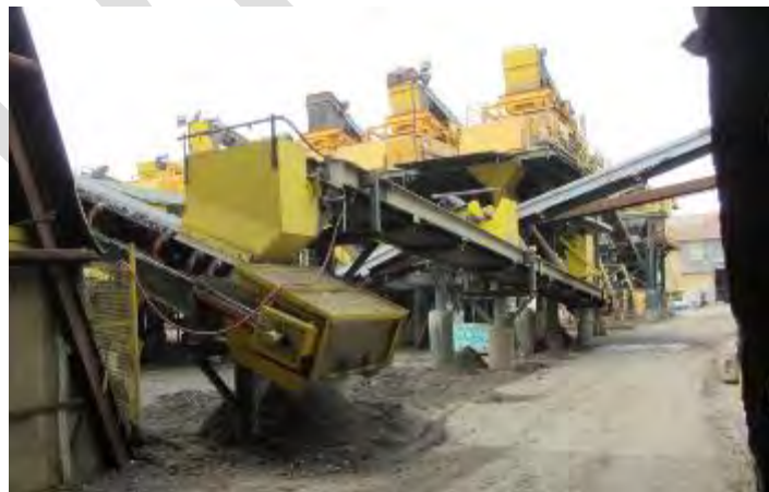
Conveyor belt lines used to transport material through the joint products plant and to the chemical treatment system at Schnitzer Steel, Inc., Oakland, CA.
