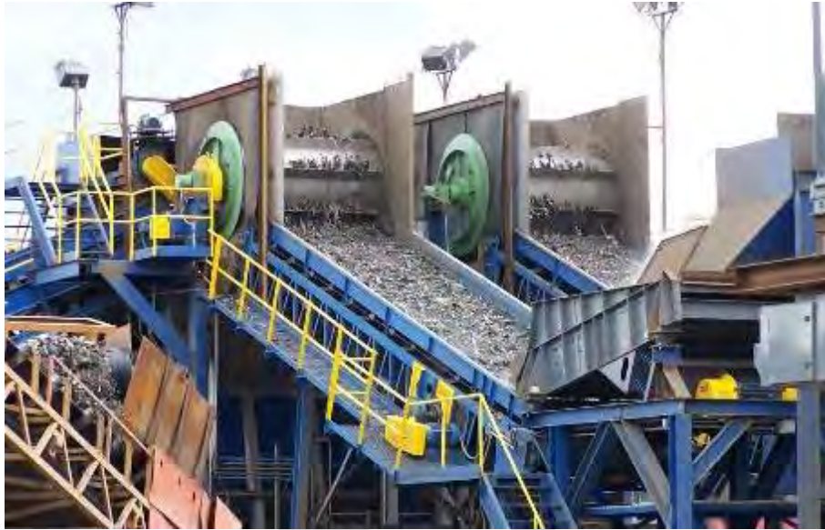
Magnets at SA Anaheim, shown here before they were enclosed.
