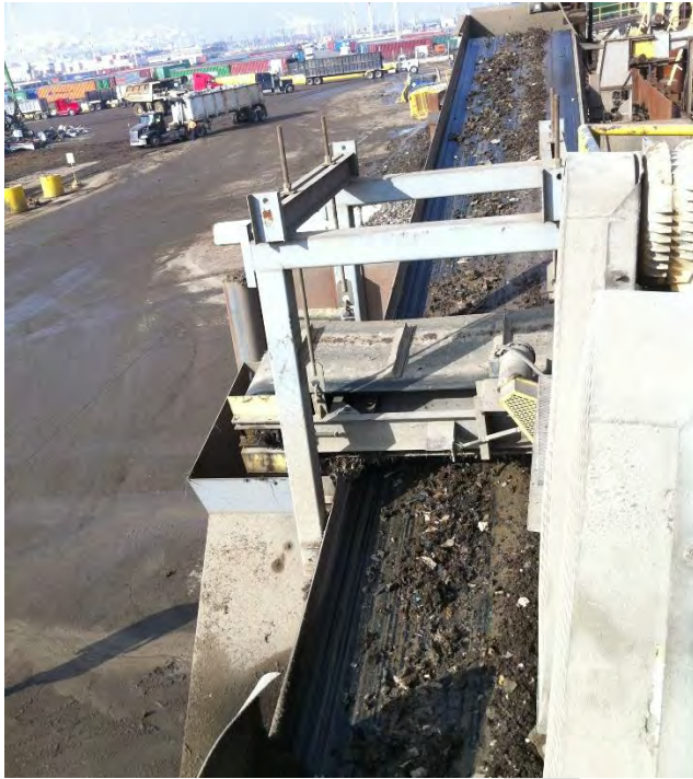
Chemically treated metal shredder residue is passed under a final magnet for recovery of ferrous metal at Schnitzer Steel, Inc., in Oakland.
