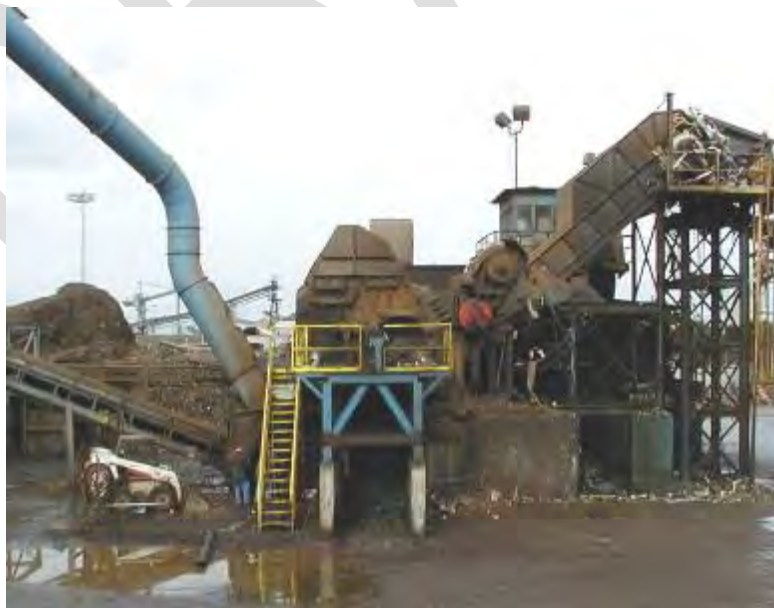
An earlier photo of the shredder unit at SA Recycling, Anaheim, CA before it was enclosed.
