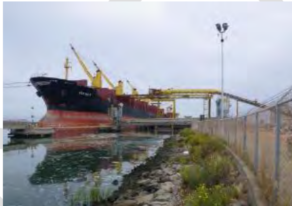
Loading sorted and shredded ferrous metals onto ship via conveyor system, Sims Metal Management, Redwood City, CA.
