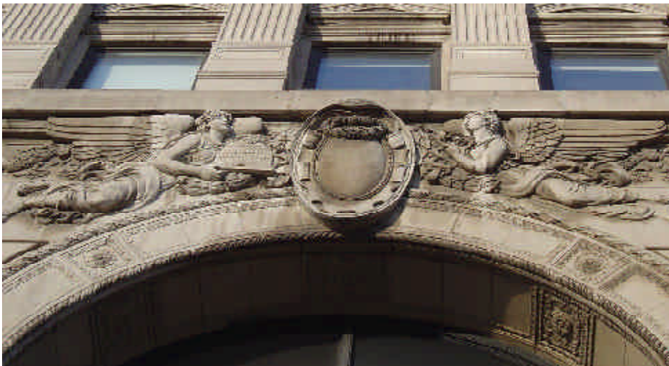
The Home Bank and Trust Company Building (commonly known as MB Financial Bank) is a six-story Classical Revival-style building. Clad with gray limestone, the building is handsomely ornamented with allegorical carved-stone figures and other Classical-style decoration.
