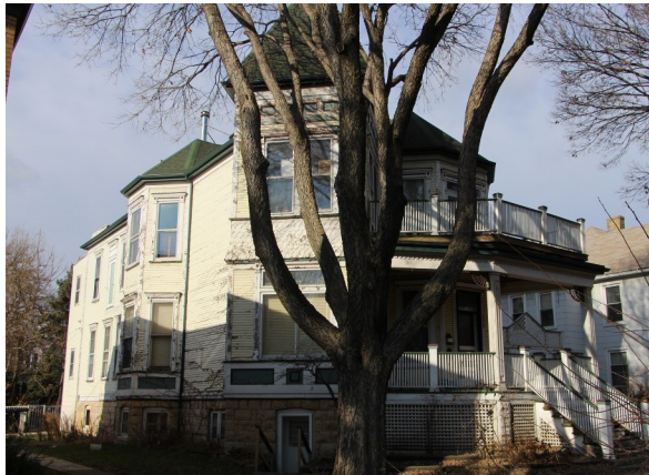
Looking down the side yard along the south elevation with its projecting bay and the buildings Joliet limestone ashlar foundation walls
