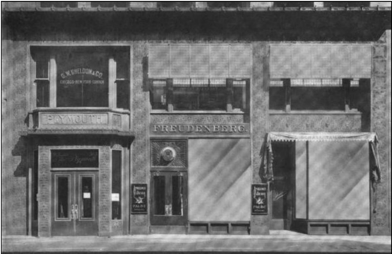
The original Dearborn Street cast iron storefront manufactured by the Winslow Brothers Company of Chicago, as seen in the company's 1901 catalog. The extant Plymouth Court cast iron storefront matches the former Dearborn Street storefront.
