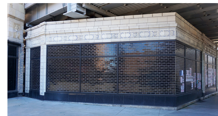
✗ Figure 41. Unacceptable example of a facadectomy as the facade has not been integrated into a new development, but left as an unoccupiable portion of a building and the storefront infilled with brick and a fake storefront frame
