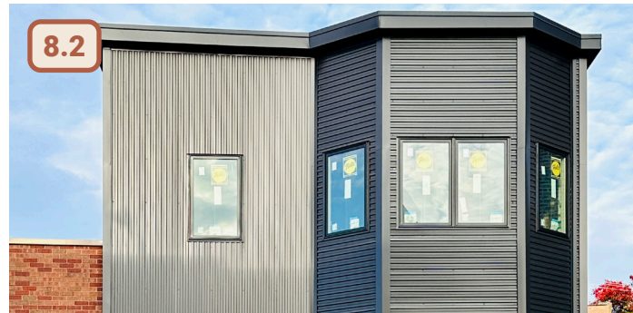
8.2 ✗ Figure 50. Unacceptable reconfiguration of upper floor window openings
