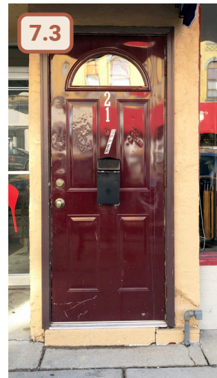
✗ Figure 47. Unacceptable example of a residential "colonial style" door
