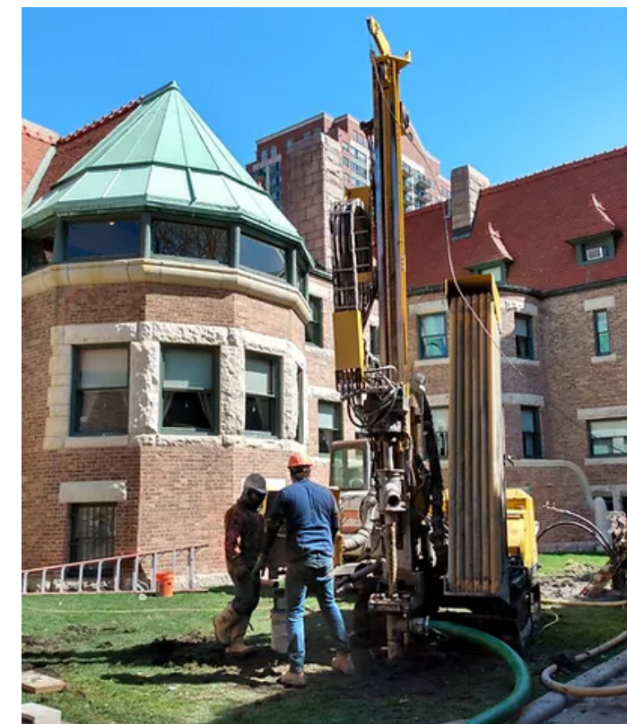
Figure 181. Example of geothermal energy being incorporated into a historic building (National Endowment for the Humanities)
