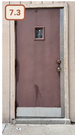
✗ Figure 46. Unacceptable example of a flush door
