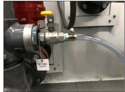
Figure 46: Effluent Sample Port
