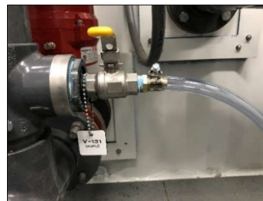
Figure 8: Pre-Treatment Sample Valve
