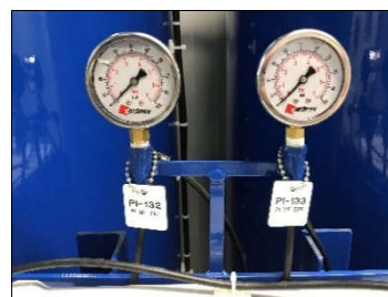
Figure 16: Media Filter Pressure Sensors
