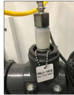
Figure 40: Treatment Polymer Injection Quill
