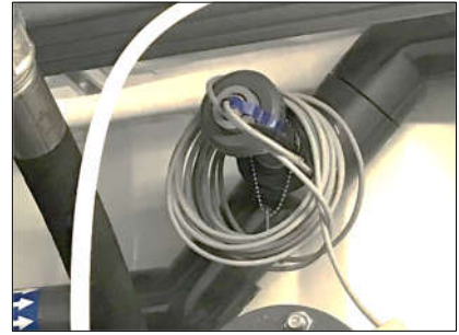
Figure 44: Treatment pH Probe
