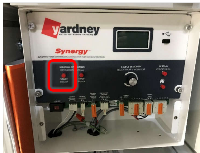
Figure 76: Media Filter Control Panel START Button
