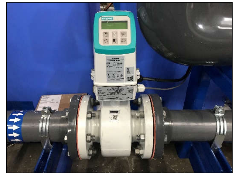
Figure 47: Effluent Flow Meter
