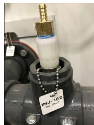
Figure 5: Caustic Injection Quill
