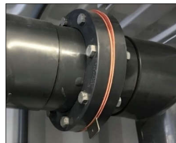
Figure 6: Pre-Treatment Plate Mixer
