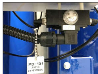
Figure 17: Media Filter Pressure Differential Indicator
