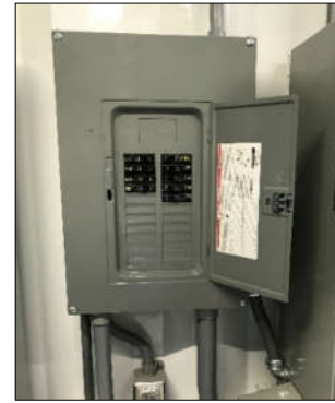
Figure 59: 120/240 V Load Center
