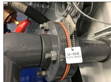
Figure 27: Post-CO 2 Injection Plate Mixer
