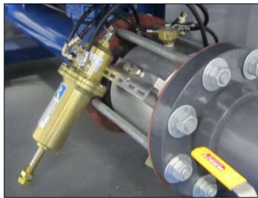
Figure 74: Example Pressure Sustaining Valve
