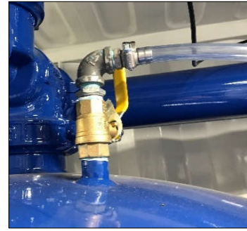
Figure 19: Media Filter Vent Valve
